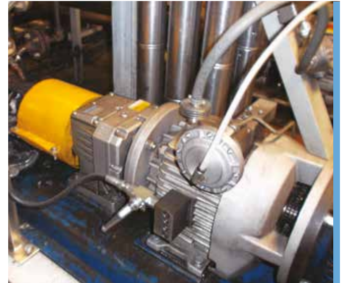
Chemical plant: K5 variator with remote pneumatic speed control.
