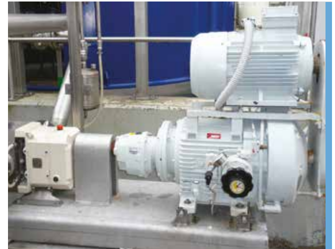
Waste treatment plant: open sky application on lobe pump, 11 kW unit with motor on top.
